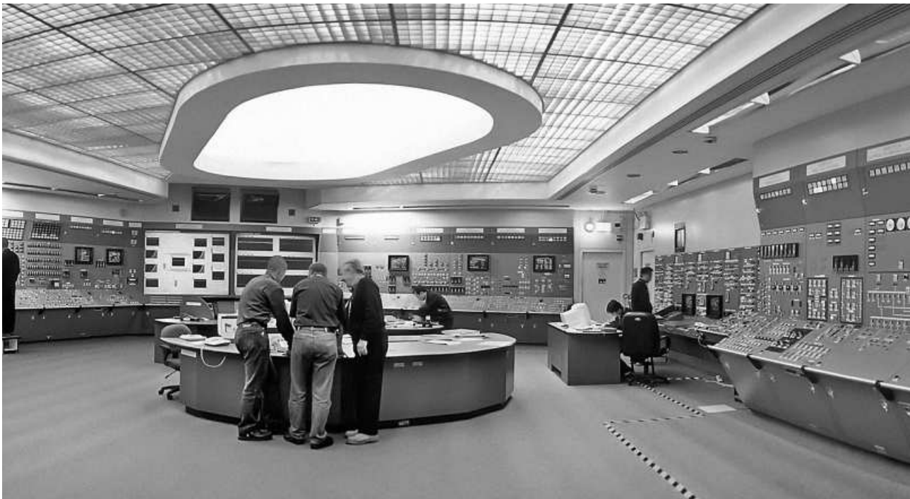
Fig. 15. CANDU-6 reactor main control room (courtesy of AECL)
